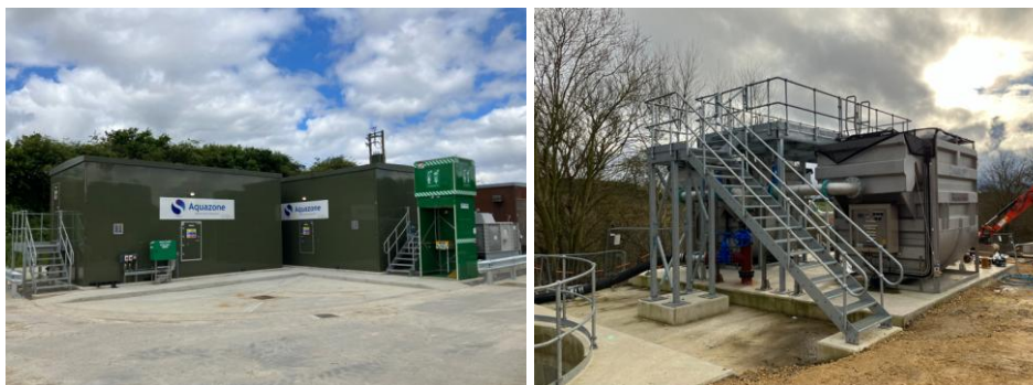
Chemical dosing kiosks containing storage tanks and dosing skids (left) and mecano for tertiary solids removal (right)
