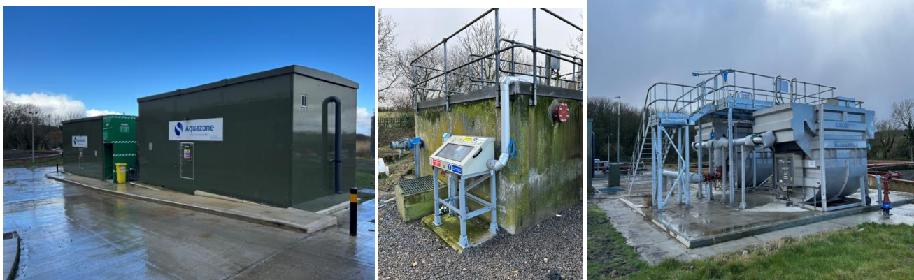
Chemical dosing equipment and Mecana installed at Sacriston STW
