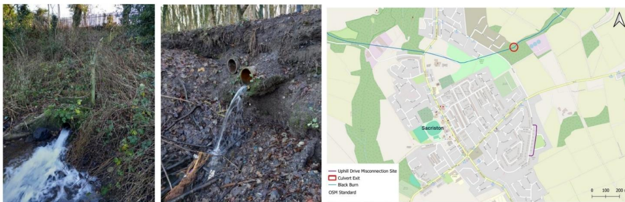
Outfall pipes from Sacriston STW (left), and from Temperley Way housing estate (centre) from where a misconnection was identified, and map showing location of pollution incident source
