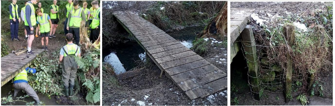
Erosion improvements on PRow bridge with volunteers
