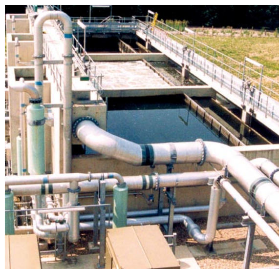
Langford water treatment works in Essex.
