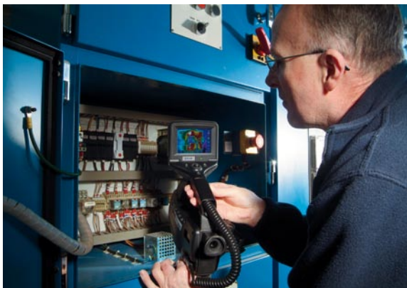
NWL's Peter Winter using a thermal imaging camera which helps to detect faults.
