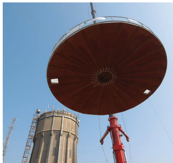
A new roof being put onto Lodgewood water tower, near Walpole in Suffolk.
