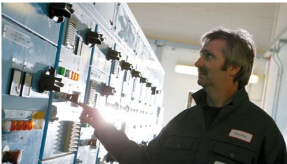
NWL's Peter Clark operating a control board at Seahouses sewage treatment works in Northumberland.
