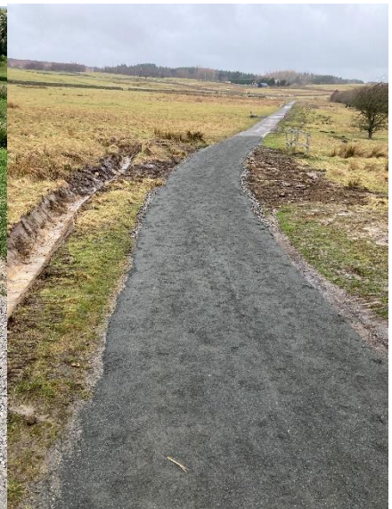
Path works after improvements: Drain relocated and path levelled out. New V ditch to effectively drain ground running towards the path
